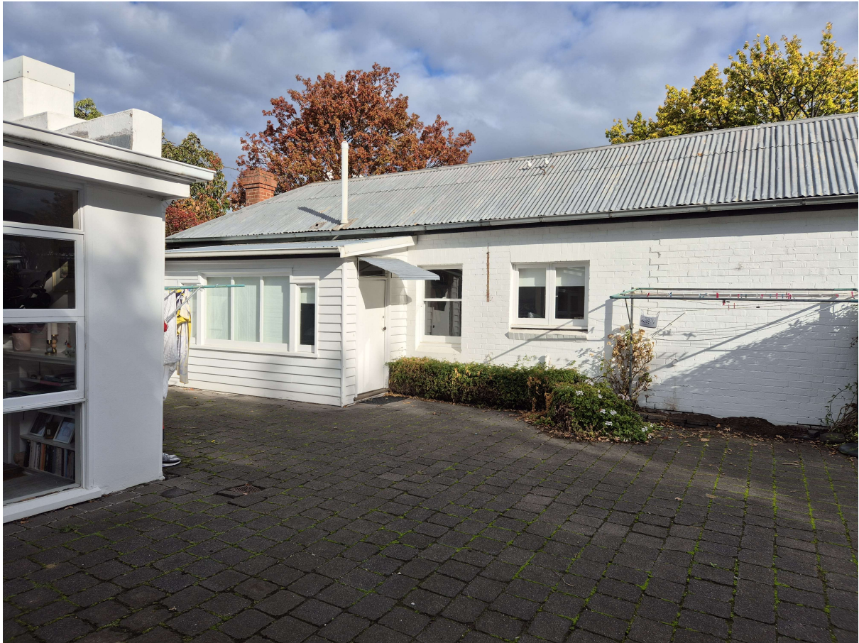
Image 6. Lean to C viewed from the back door of the existing dwelling. Refer to demolition plan for the location of image6.
