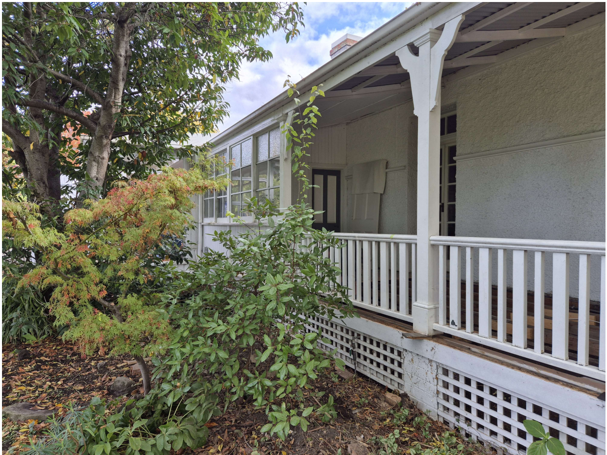
Image 3. Lean to B viewed from the North East garden. Note the timber brackets on the existing verandah posts to be replicated. Refer to the demolition plan for the location of image 3.
