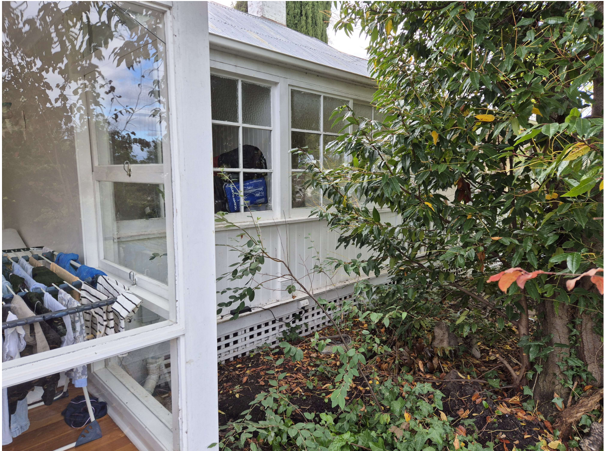
Image 4. Lean to B viewed from the South East Garden. Note the existing, original verandah post that will be retained, made good, and restored to match the original verandah posts. Refer to the demolition plan for the location of image 4.
