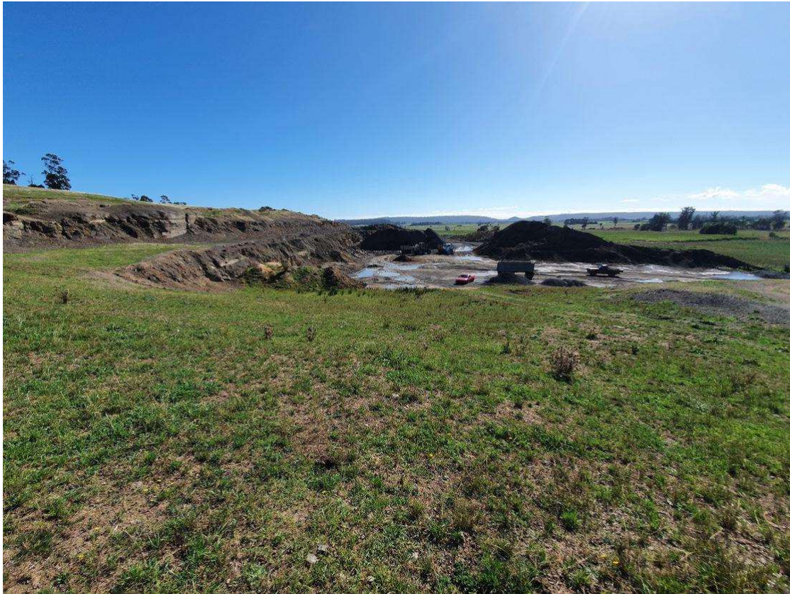
Figure 17. Rehabilitation of previously disturbed area (foreground) and active quarry area (background), facing north.
