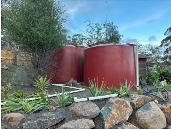
Existing tank may provide the required static Firefighting water supply. Protection by shielding of the tank itself and the material on the bottom 400mm of tank is required
