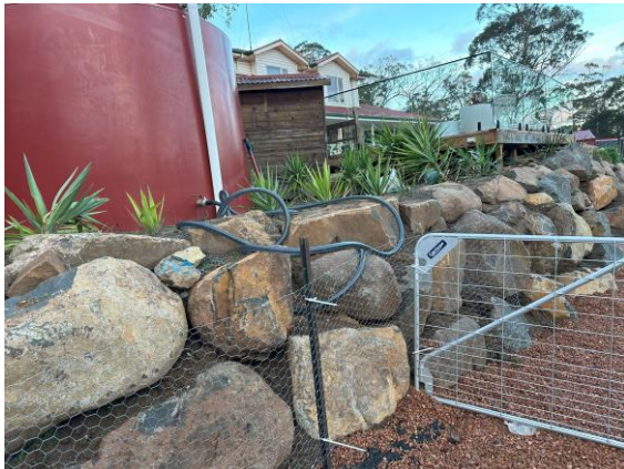
Signage of the firefighting water tank is required
