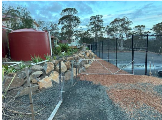
Hardstand area for tank which is likely to provide static firefighting water supply (tank will need to be upgraded to comply)
