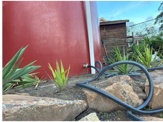
Fixtures & fittings need to comply with DD requirements
