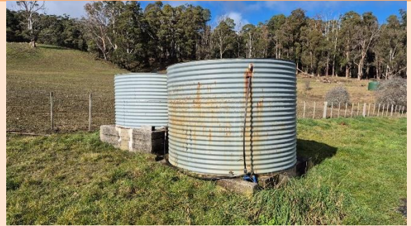
Existing metal water tanks – non-compliant for fire fighting purposes due to less than 10,000l
