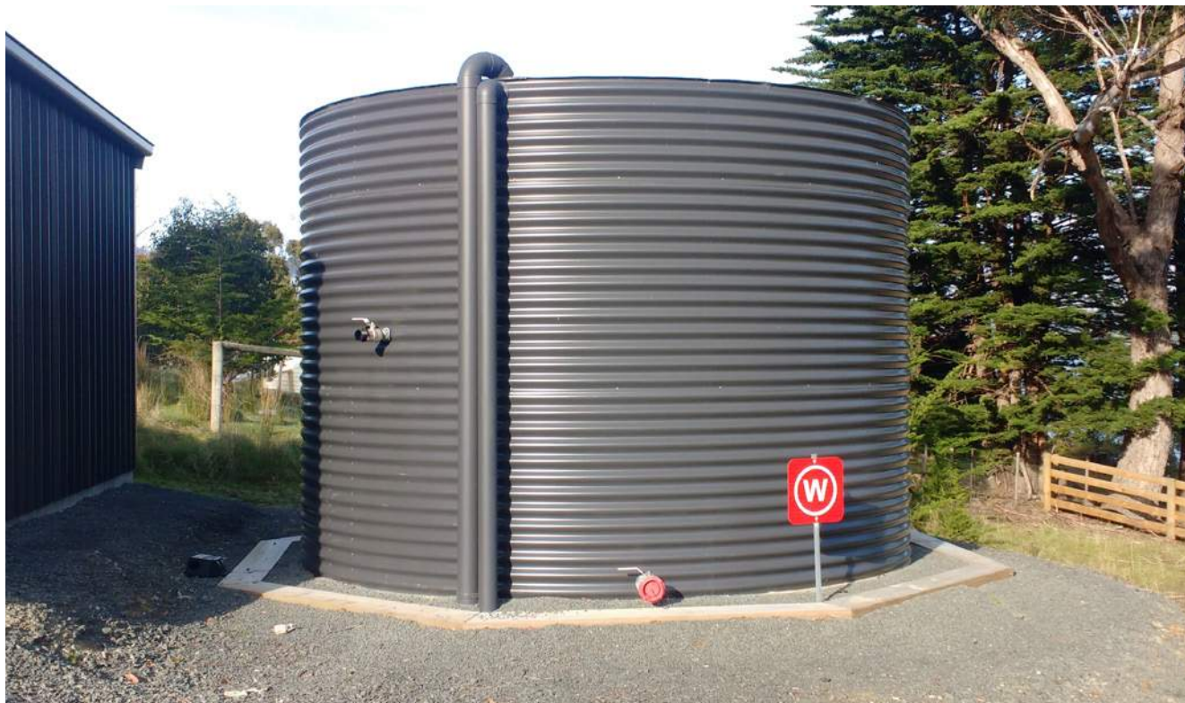
Figure 2 An example of a compliant combination static supply where the bottom 10,000 litres is reserved for firefighting purposes and the remainder is available for domestic use by the property owner.
