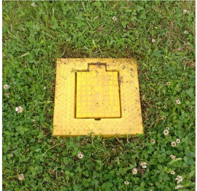
Figure 8 An image of a suburban hydrant cover plate under which is located a ground ball hydrant
