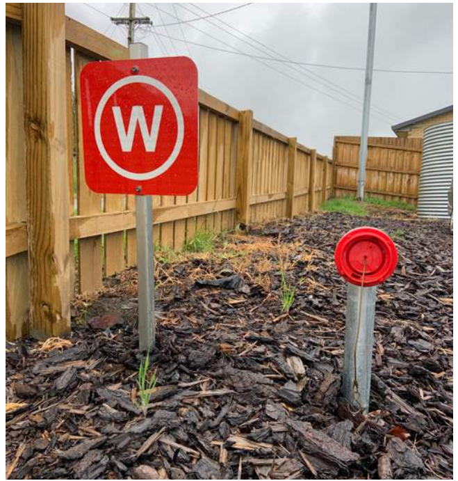
Figure 4 Shows a compliant example of a remote take-off from the 10,000 litre firefighting water supply tank.
