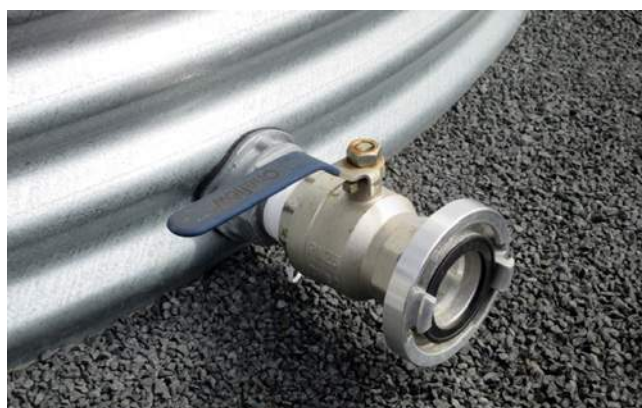
Figure 3 Shows a Storz coupling fitted to a static water supply.
