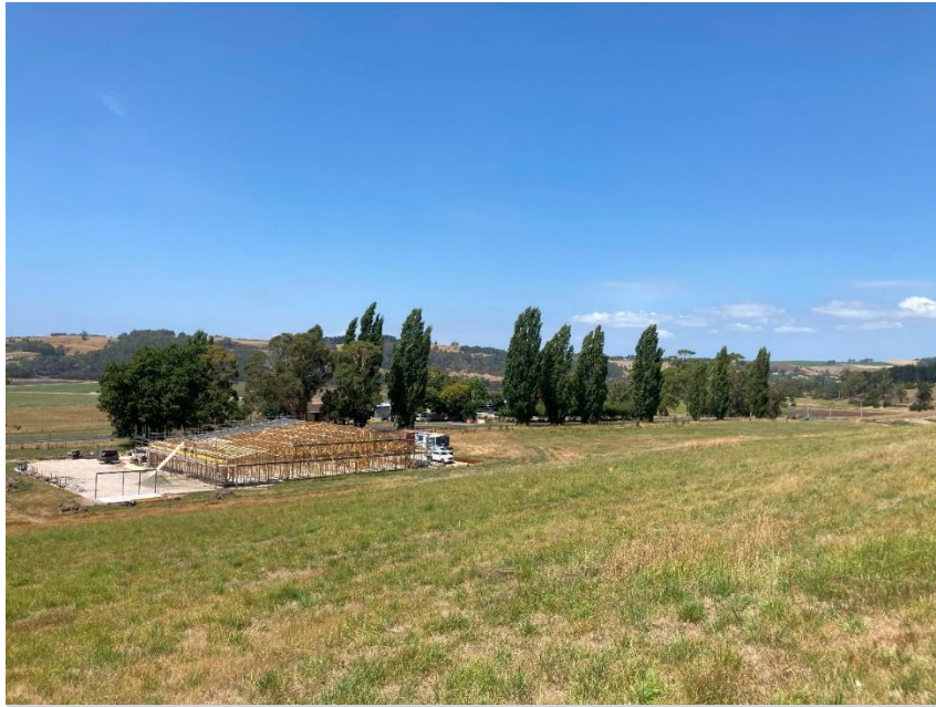
Figure 11 Veterinary clinic under construction, showing some existing vegetation buffering between the clinic and neighbouring residential dwellings.
