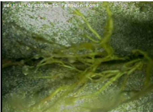
19, 00:13:59, 22.83 Recently cut fine roots—a relatively small number of cut minor roots remain, Obstruction: 10%, at joint from 9 o'clock to 11 o'clock
