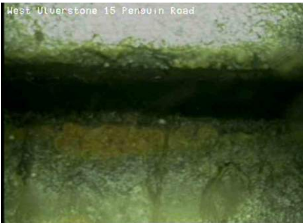
23, 00:16:36, 26.54 Joint displaced longitudinal, 10mm
