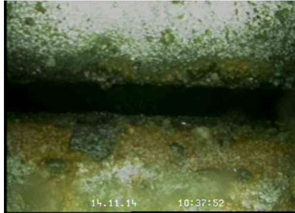
18, 00:13:05, 21.58 Joint displaced longitudinally, 10mm
