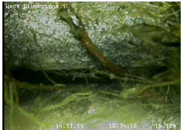
12, 00:10:25, 19.12 Recently cut fine roots—a relatively small number of cut minor roots remain, Obstruction: 10%, at joint from 8 o'clock to 10 o'clock
