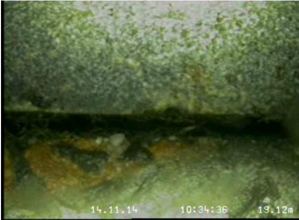
13, 00:10:40, 19.12 Joint displaced angular at 12 o'clock
