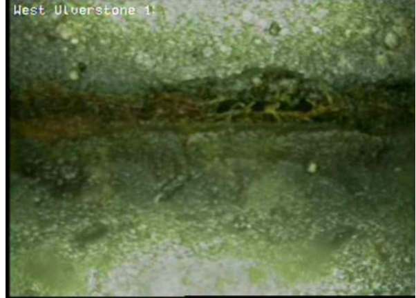
6, 00:05:07, 9.31 Recently cut fine roots—a relatively small number of cut minor roots remain, Obstruction: <5%, at joint from 8 o'clock to 4 o'clock
