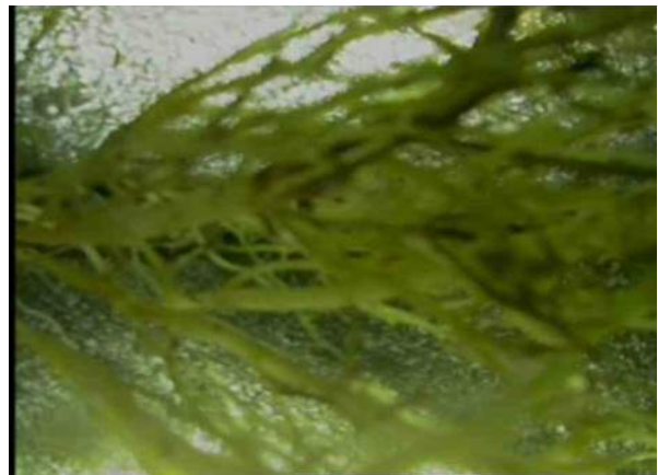
24, 00:16:47, 26.54 Recently cut fine roots—a relatively small number of cut minor roots remain, Obstruction: 10%, at joint from 2 o'clock to 4 o'clock
