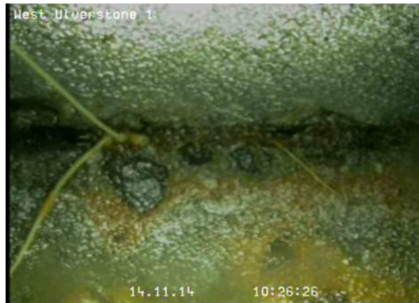
4, 00:03:47, 6.83 Recently cut fine roots—a relatively small number of cut minor roots remain, Obstruction: <5%, at joint from 9 o'clock to 10 o'clock
