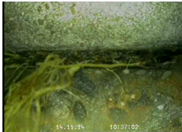
16, 00:12:38, 21.58 Recently cut fine roots—a relatively small number of cut minor roots remain, Obstruction: 10%, at joint from 8 o'clock to 10 o'clock
