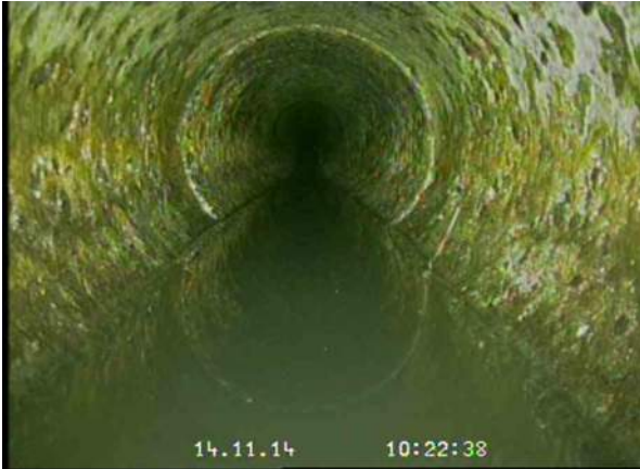
1, 00:00:28, 0.13 Ponding of water with or without flow turbid or discoloured water, 10-20 mm
