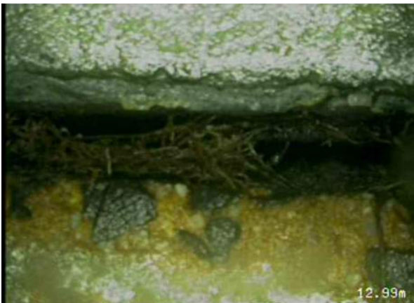
11, 00:07:59, 12.99 Joint displaced longitudinally, 10mm
