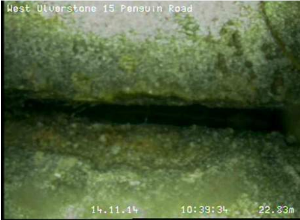
21, 00:14:22, 22.83 Joint displaced angular at 1 o'clock
