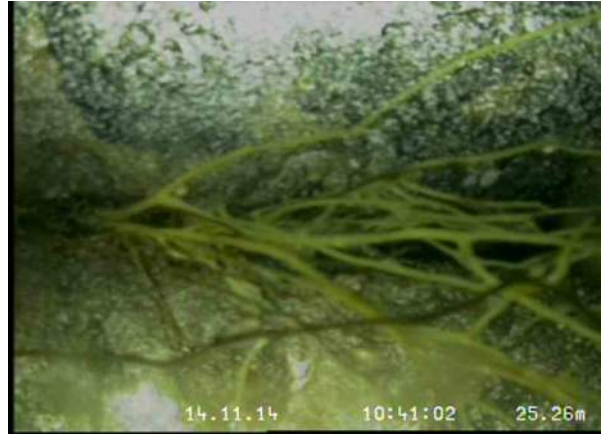
22, 00:15:42, 25.26 Recently cut fine roots—a relatively small number of cut minor roots remain, Obstruction: 10%, at joint from 8 o'clock to 4 o'clock
