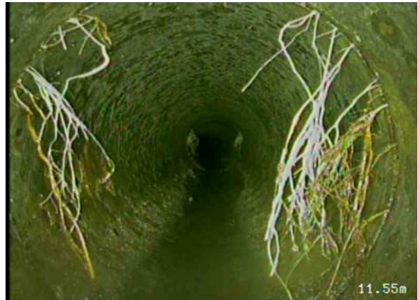
8, 00:06:31, 11.55 Recently cut fine roots—a relatively small number of cut minor roots remain, Obstruction: 10%, at joint from 8 o'clock to 4 o'clock
