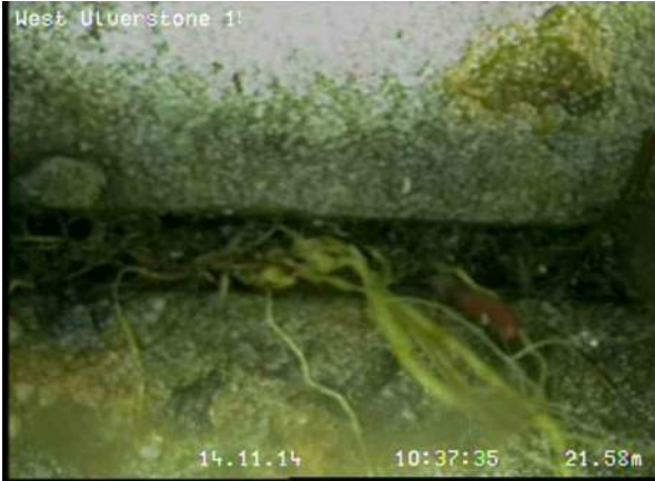
17, 00:12:55, 21.58 Recently cut fine roots—a relatively small number of cut minor roots remain, Obstruction: 10%, at joint from 3 o'clock to 4 o'clock
