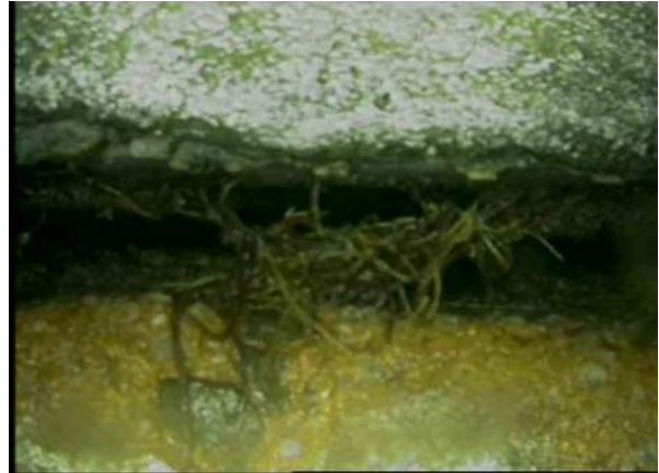
10, 00:07:50, 12.99 Recently cut fine roots—a relatively small number of cut minor roots remain, Obstruction: 10%, at joint from 8 o'clock to 4 o'clock
