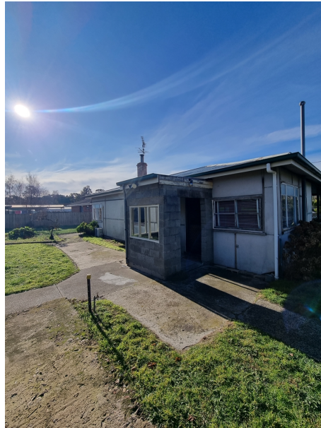
Figure 2. A small lean-to structure sits underneath the existing eaves at the dwelling's entry; its lack of reinforced structure and waterproofing neglect runs risks of damaging both the main dwelling and occupant. This structure is not believed to be of the original dwelling's construction
