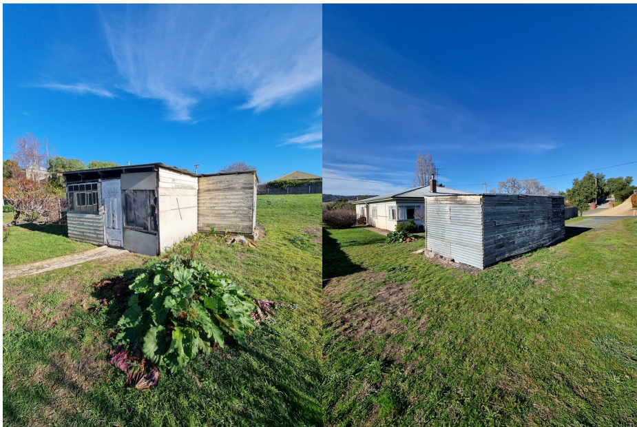
Figure 3. The conjoined outbuildings were once used as a shed and carport, both structures are finished with a range of adhoc materials which are currently falling apart. Both structures have fallen into disrepair.
