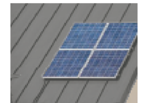
MR.01 - Metal Deck Roof PV Panels
