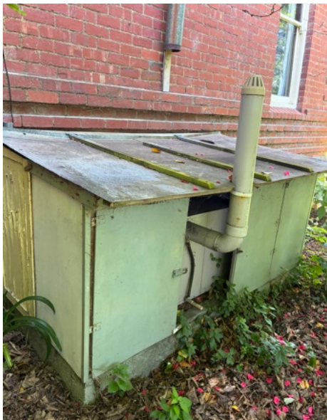
Existing heating system to be removed on southern edge of house. Fabric of low significance.
