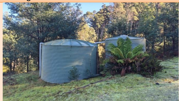
Existing poly tanks – Lot 2 (non-compliant for fire fighting purposes due to material)
