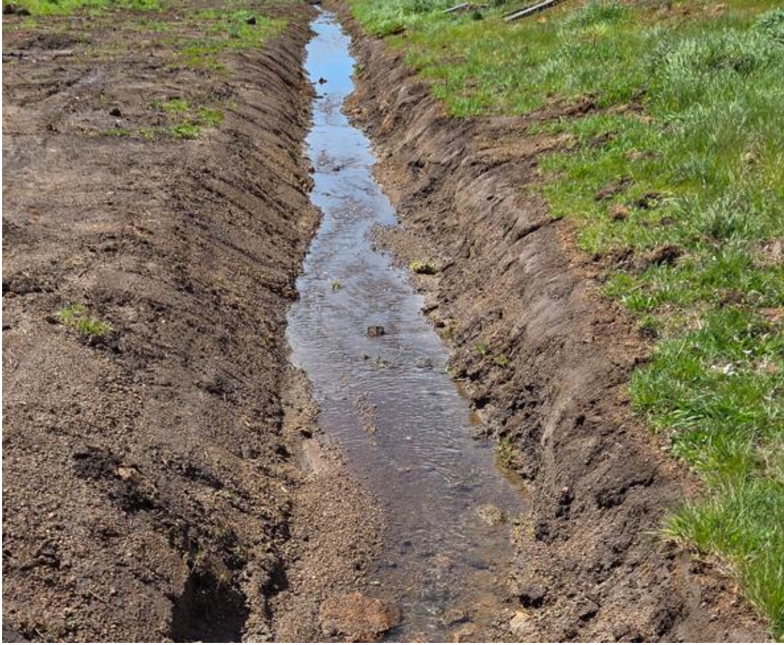
Figure 8 Southern drain typical construction. Note it has just been cleaned out hence lack of vegetation on banks
