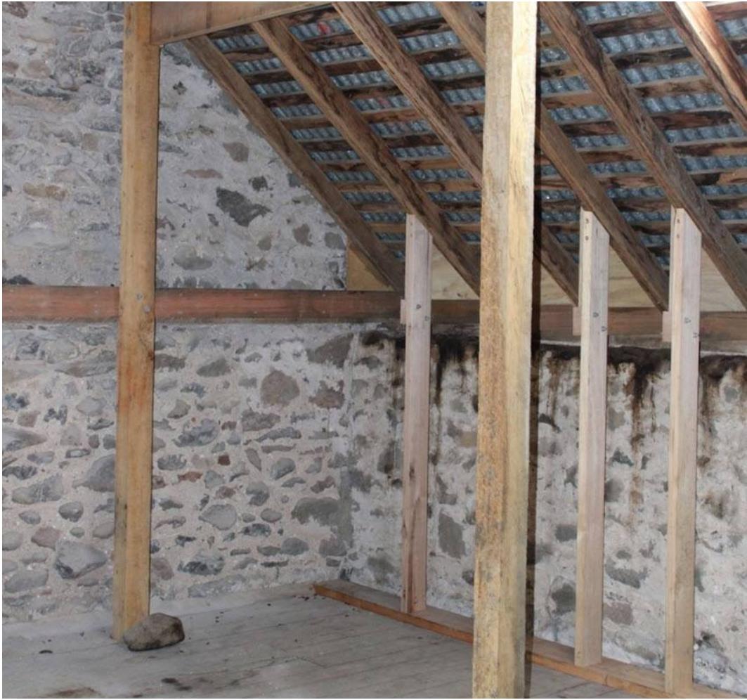
Figure 4: Interior of first floor showing timber roof and flooring construction with stone walls
