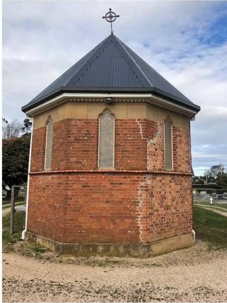
West end of the church showing bayed end hipped roof and more recent restoration work
